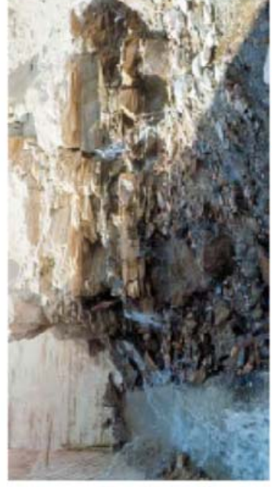
Fontenelle Dam Incident, Wyoming, USA from USBR
